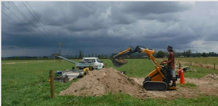
Figure 1: Tasman McKelvey operates the skid steer loader at the denitrifying bioreactor site.
